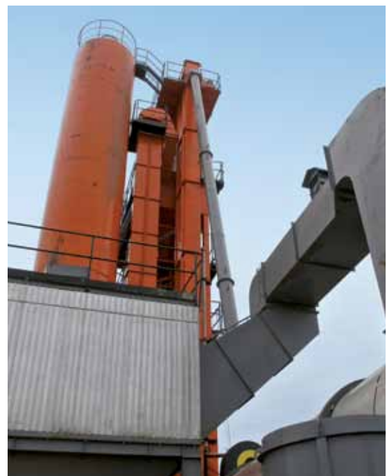
Filtering system in an asphalt production plant
