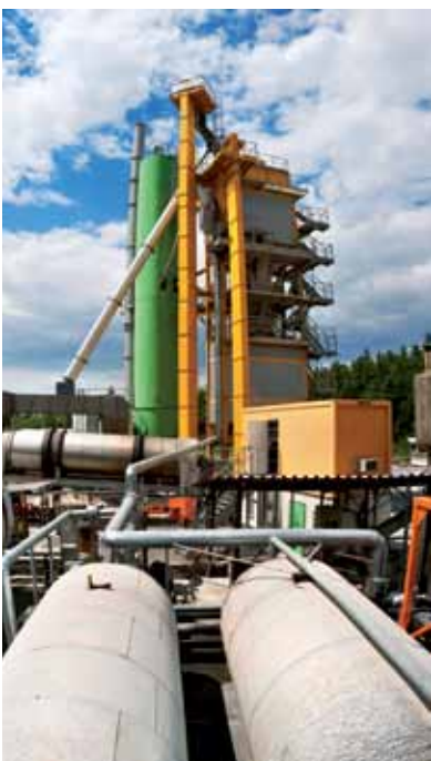
Asphalt production plant
